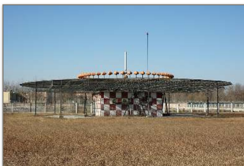
A DVOR station
